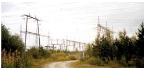
Figure 3. A photo from outside of the substation.
